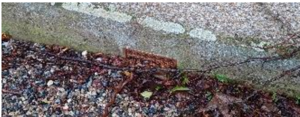
The air brick at this farmhouse near Stoke Climsland is partially covered by the external surfacing which could be restricting air flow under timber floors.
