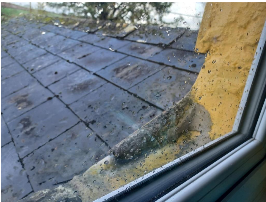
The cill at this house near Downgate is lipped at one end and could be potentially trapping water.
